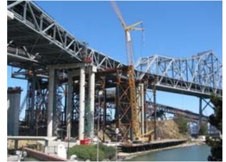
An EarthCam camera view of San Francisco Bay Bridge seismic retrofit project
